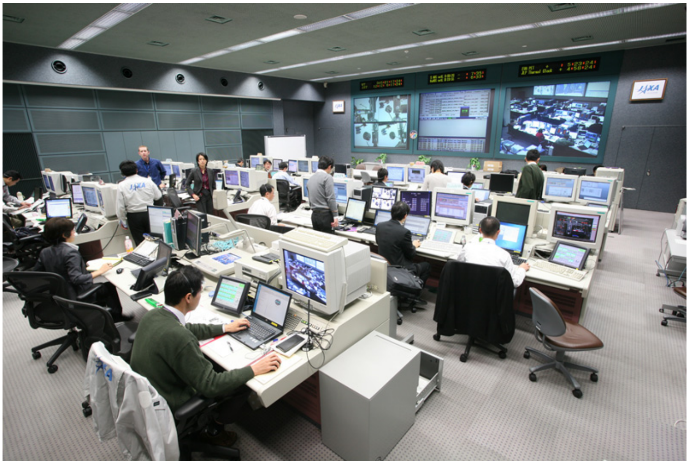
Kibo Mission Control Room
